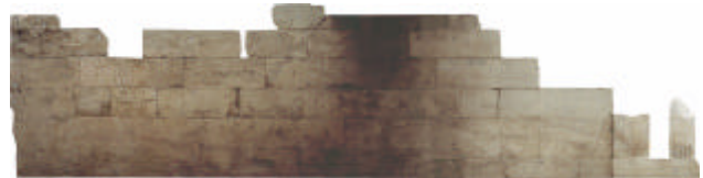
Figure 5. Three meters high corridor. The dark part was under shadow and processed with wallis filtering, prior to mosaicking.
